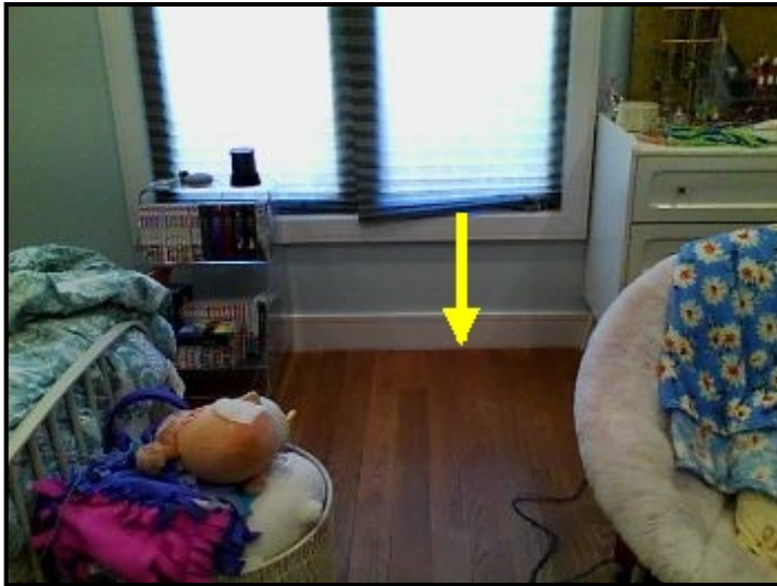
Water entry into lower wall area.
