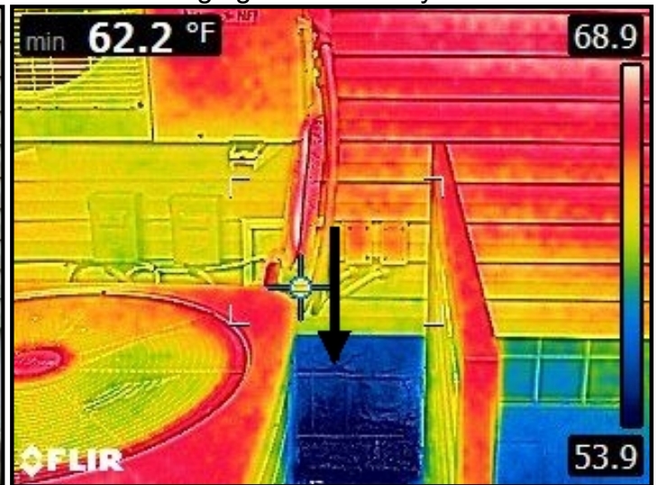
Infrared imaging of water entering through siding around utility connection points and cascading down into the internal wall areas below.
