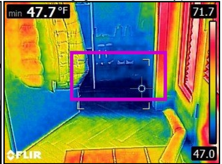
Infrared imaging of severe draft entry point.
