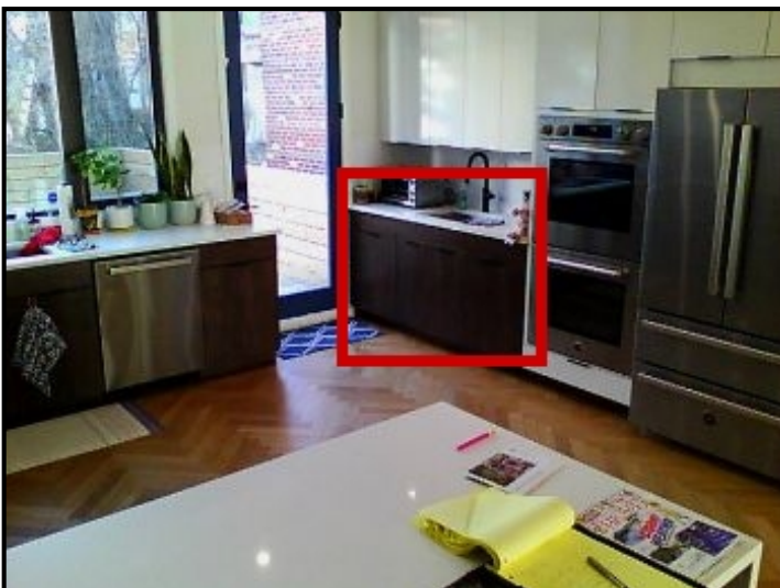
Repair Point: Remove cabinets from wall area. Excavate drywall. Install proper insulation.
