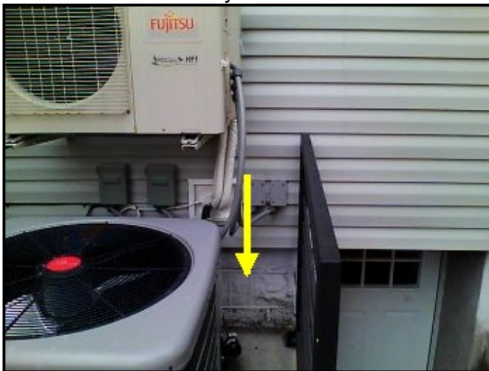
Water entering through siding around utility connection points and cascading down into the internal wall areas below.
