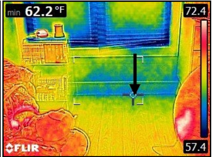
Infrared imaging of water entry into lower wall area.
