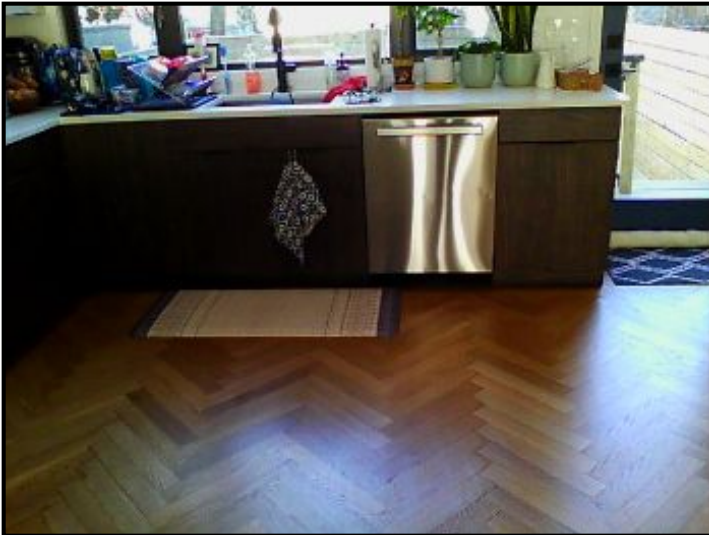
Severe draft entry point.
