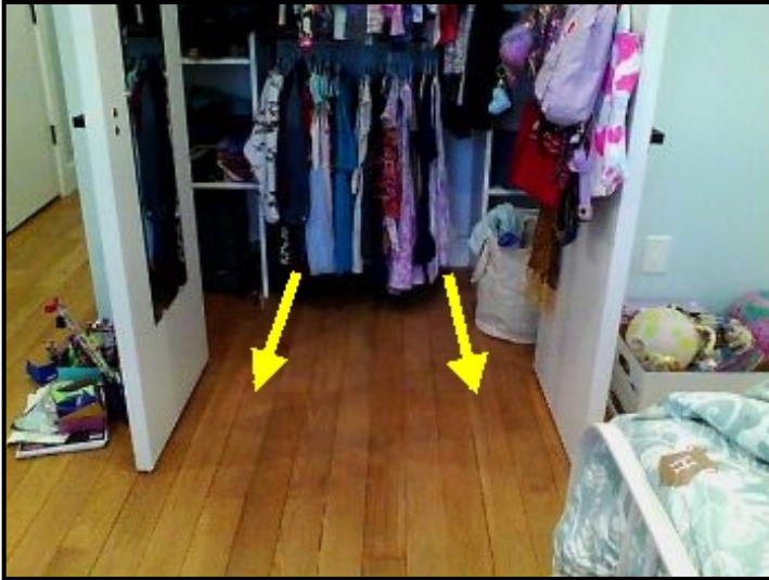
Water entry point into closet wall area.
