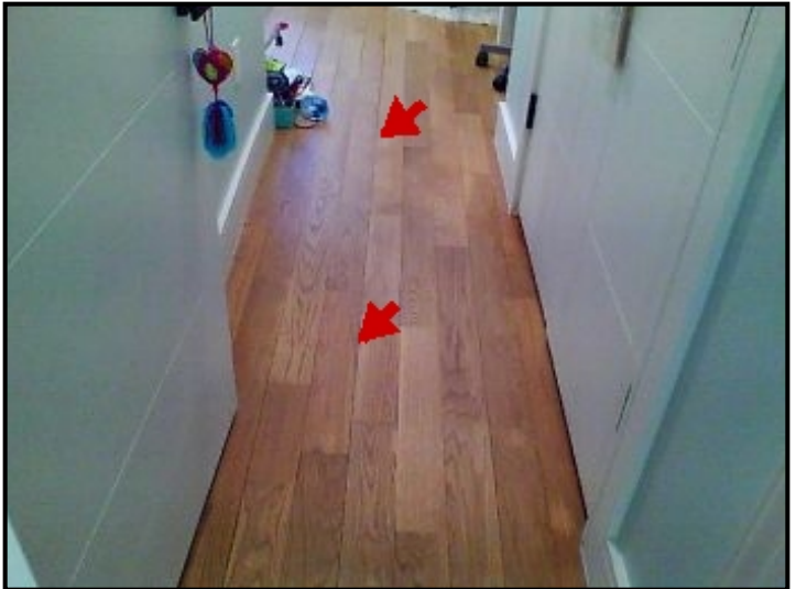
Repair Point: Conduct followup scans to confirm findings. If confirmed, replace floor boards.
