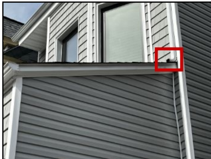
Repair Point: Route gutter leader away from roof edge.
