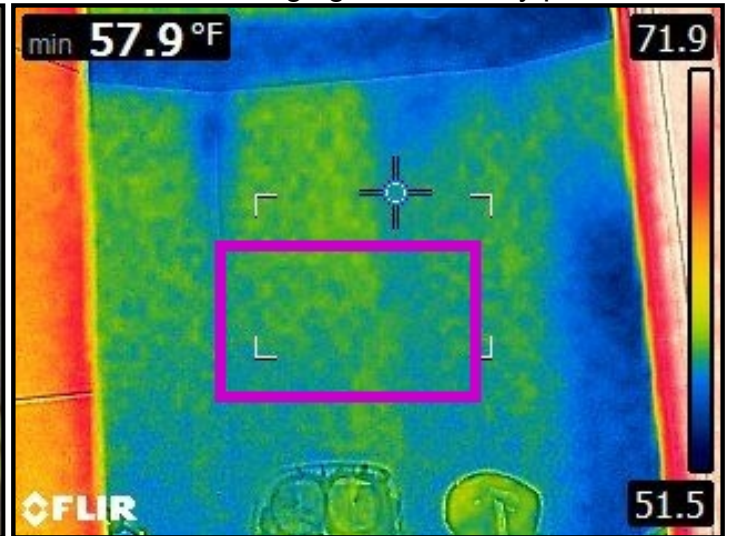
Infrared imaging of draft entry point.
