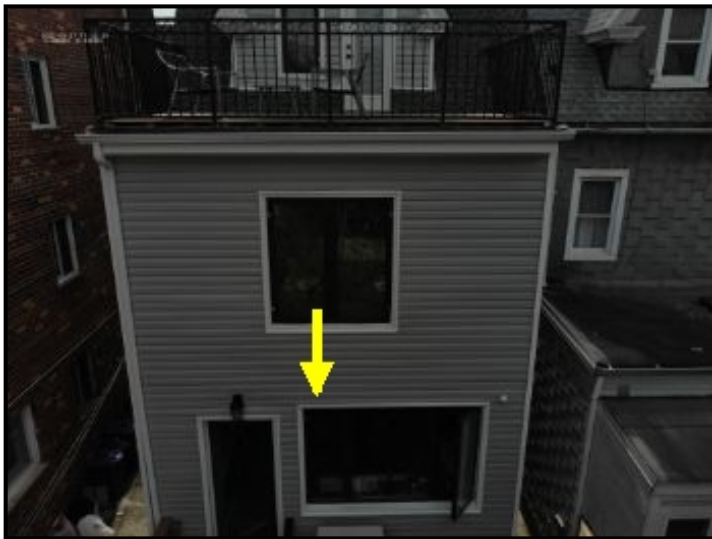
Water entering through window sill connection point to facade and backflowing into the internal wall area.
