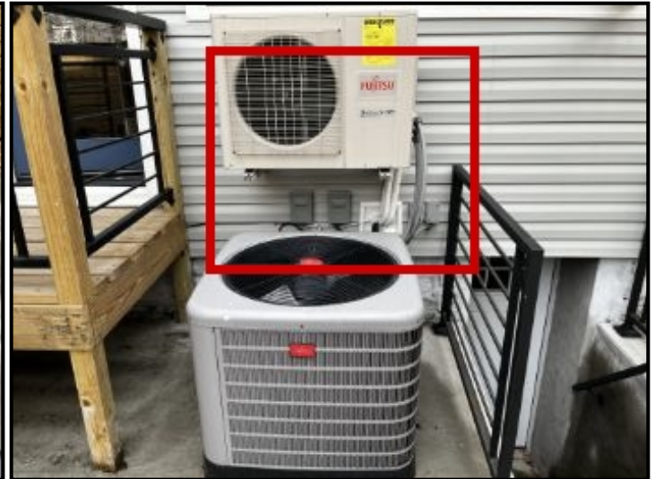
Repair Point: Seal around air handler bracket anchor points and around electrical utility connection points to facade.
