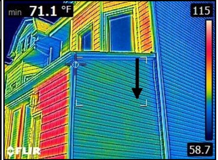
Infrared imaging of water entry into side facade from above gutter leader deposit point draining into the roof substrate and depositing into the side facade.
