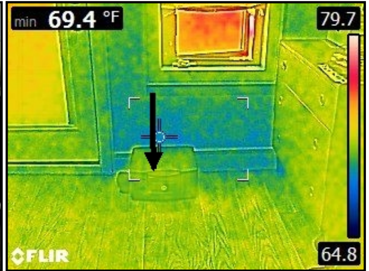
Infrared imaging of water entering into wall area and cascading down into the second floor closet floor area.
