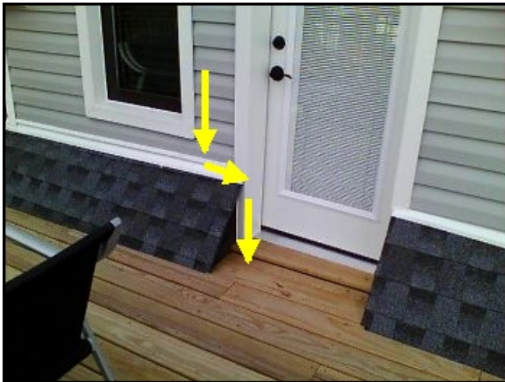
Water entering through facade area, backflowing into the internal wall and cascading down into the second floor closet floor area.
