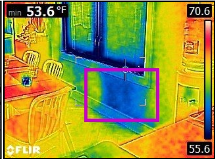
Infrared imaging of draft entry point.
