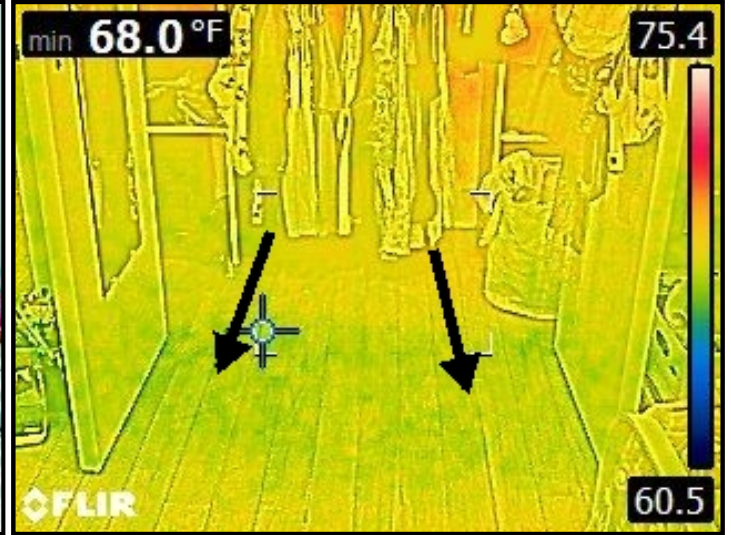
Infrared imaging of water entry point into closet wall area.
