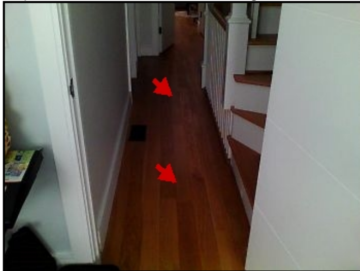
Repair Point: Conduct followup scans to confirm findings. If confirmed, replace floor boards.
