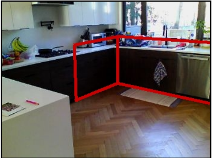
Repair Point: Remove cabinets from wall area. Excavate drywall. Install proper insulation.
