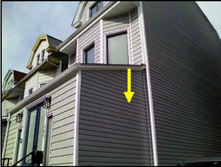
Water entry into side facade from above gutter leader deposit point draining into the roof substrate and depositing into the side facade.
