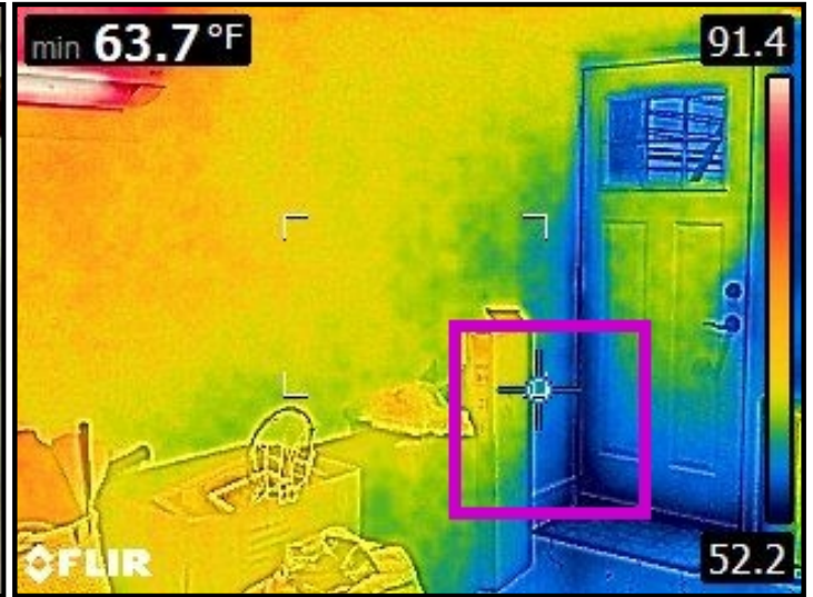
Infrared imaging of draft entry point.
