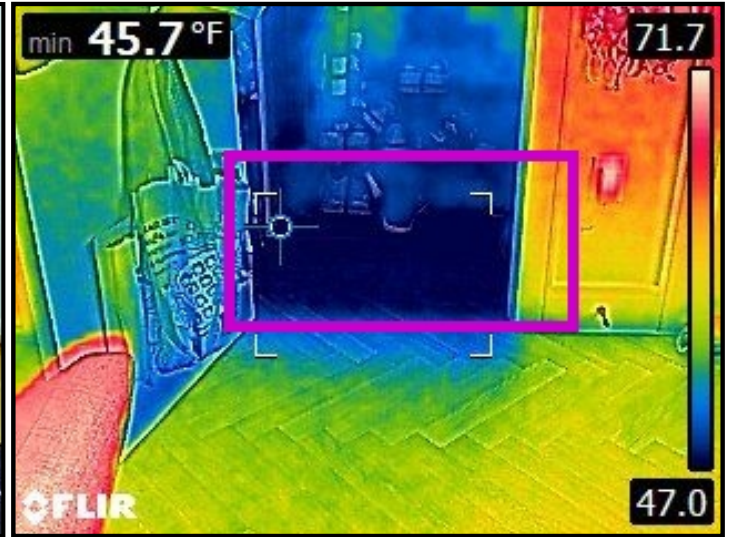
Infrared imaging of severe draft entry point.
