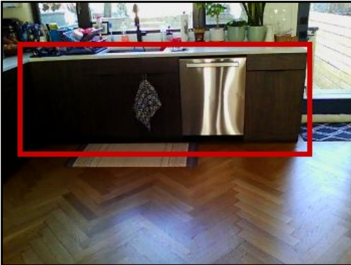
Repair Point: Remove cabinets from wall area. Excavate drywall. Install proper insulation.
