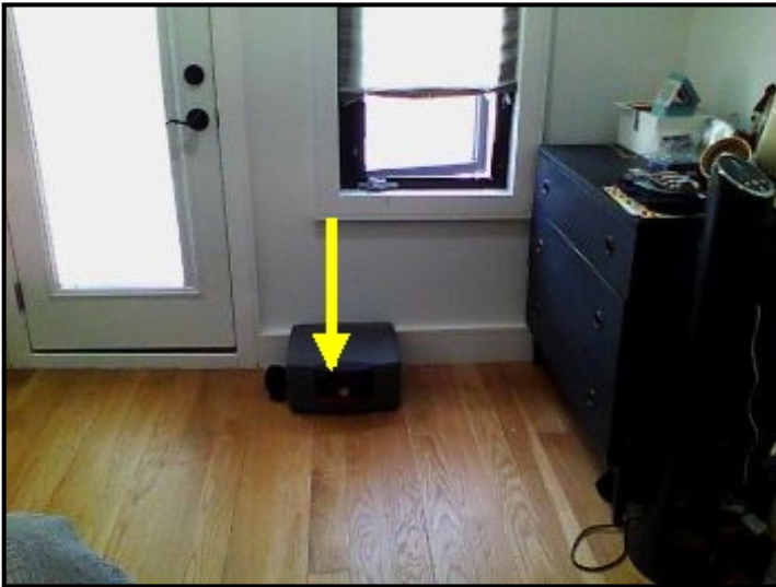
Water entering into wall area and cascading down into the second floor closet floor area.
