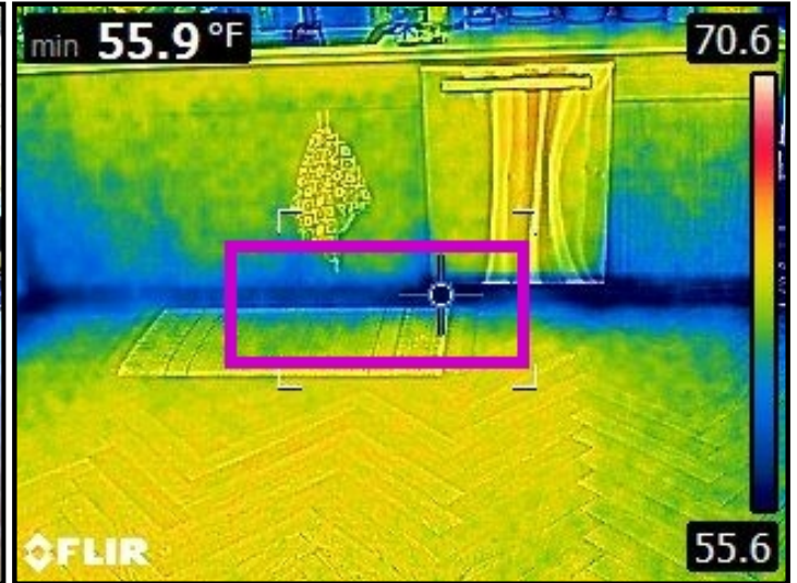
Infrared imaging of severe draft entry point.
