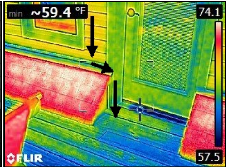
Infrared imaging of water entering through facade area, backflowing into the internal wall and cascading down into the second floor closet floor area.
