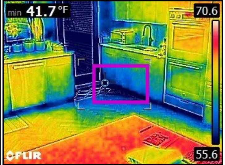
Infrared imaging of severe draft entry point.
