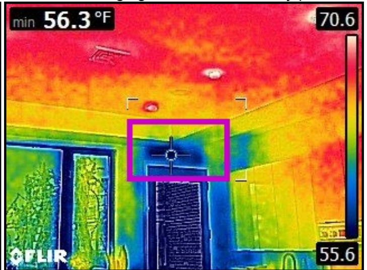
Infrared imaging of severe draft entry point.
