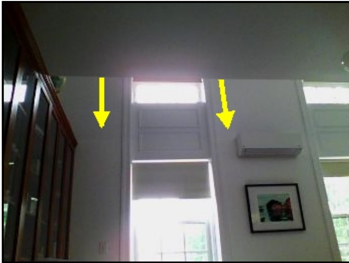
Water entry into wall area.
