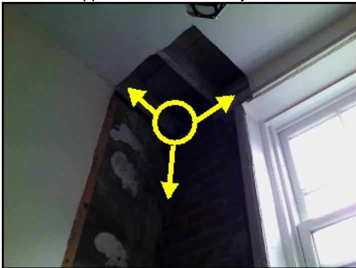
Severe water entry into corner wall area from upper roof membrane system.
