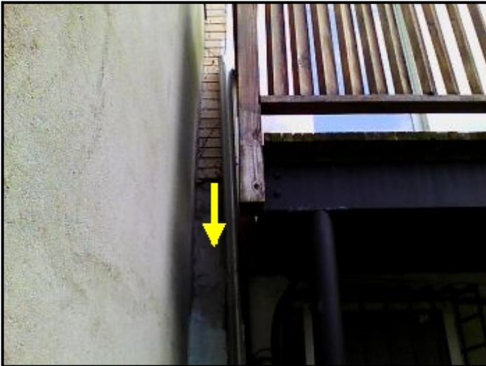
Water entering through rear facade and backflowing into the internal wall area.
