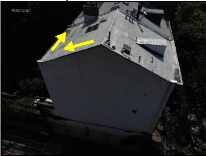
Water entering through roof membrane system connection point to the coping stone and cascading down into the rear facade.
