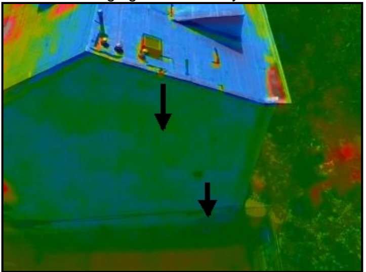
Infrared imaging of water entering through roof membrane/parapet wall coping stone connection point, cascading down through the side facade and depositing into the internal wall areas below.
