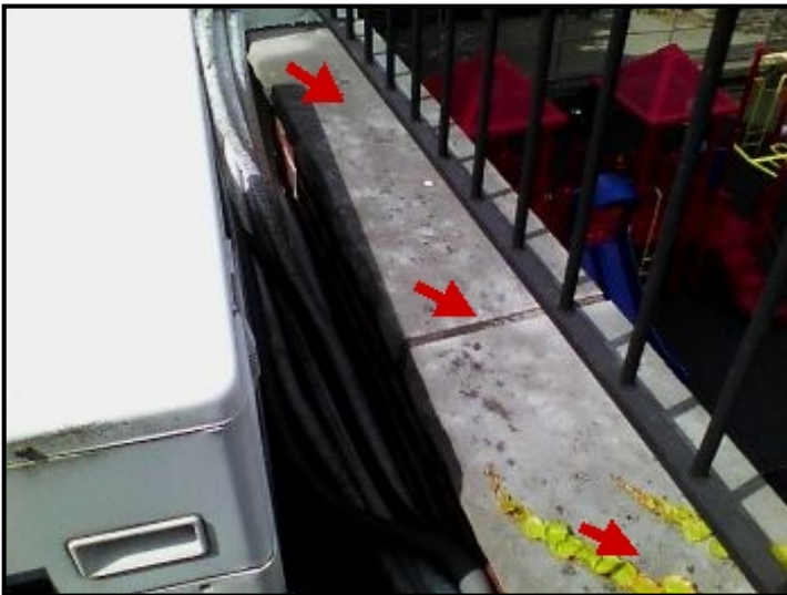
Repair Point: Waterproof parapet wall brick. Install aluminum flashing cap over parapet coping stone. Seal outer brick.
