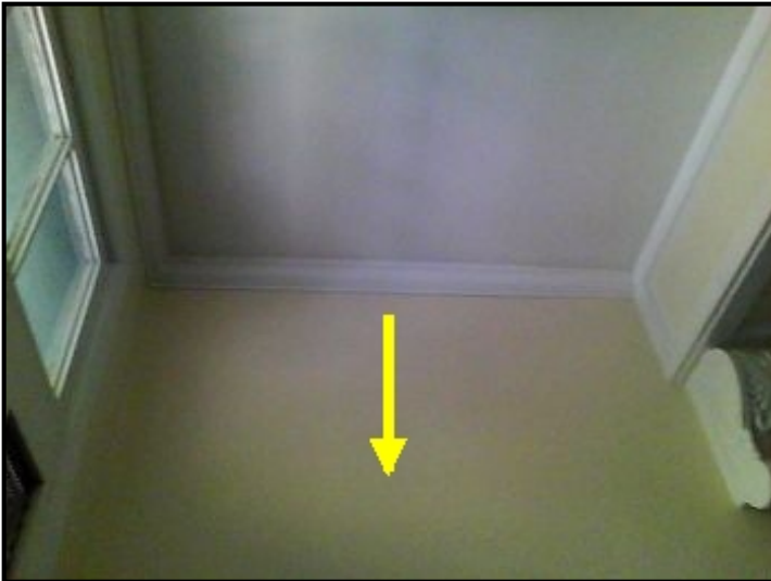
Water entry into wall area.
