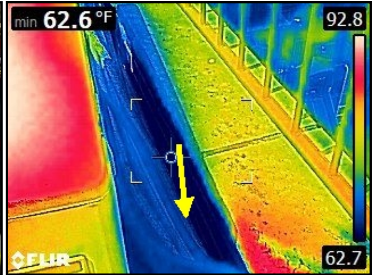
Infrared imaging of water entering through parapet wall coping stone system and cascading down into the ceiling/wall area below.
