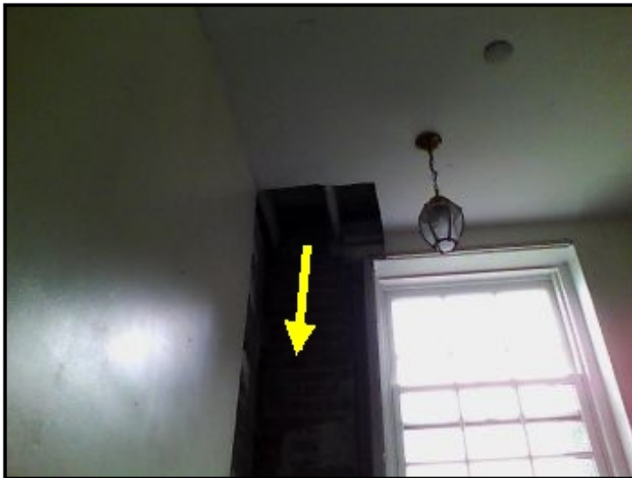
Severe water entry into corner wall area from upper roof membrane system.
