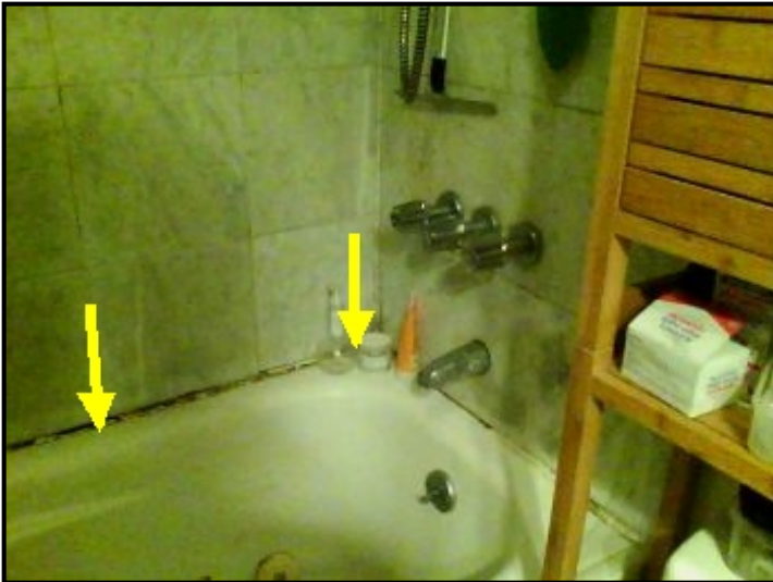
Water entering through shower stall tile wall area and cascading down into the ceiling area below.
