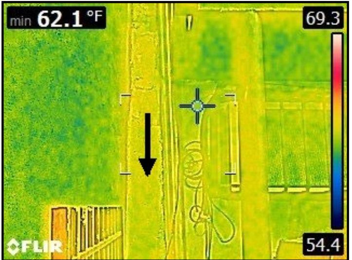
Infrared imaging of water entering through rear facade and backflowing into the internal wall area.
