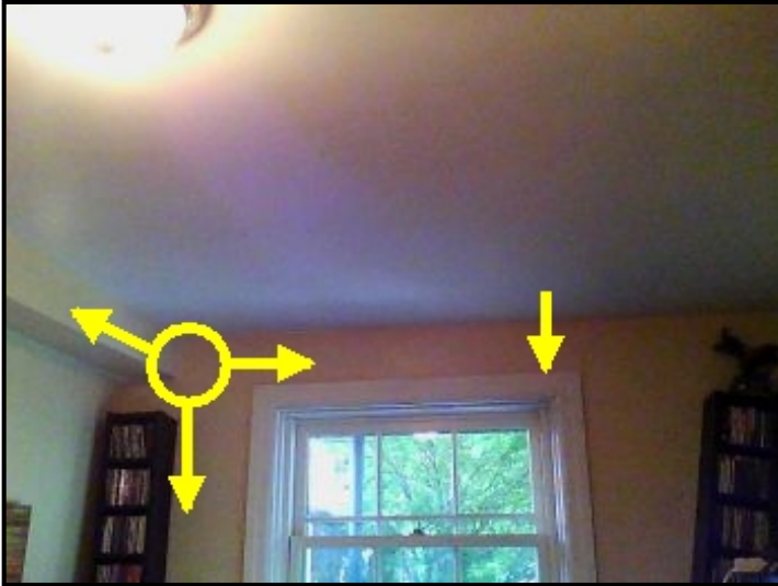
Water entry into wall/ceiling area.
