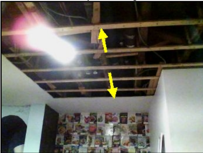
Water entry into ceiling area.
