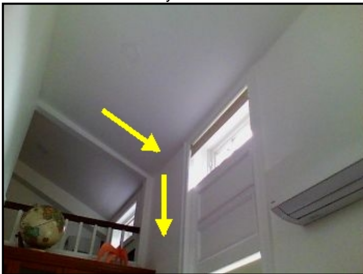
Water entry into ceiling/wall area.
