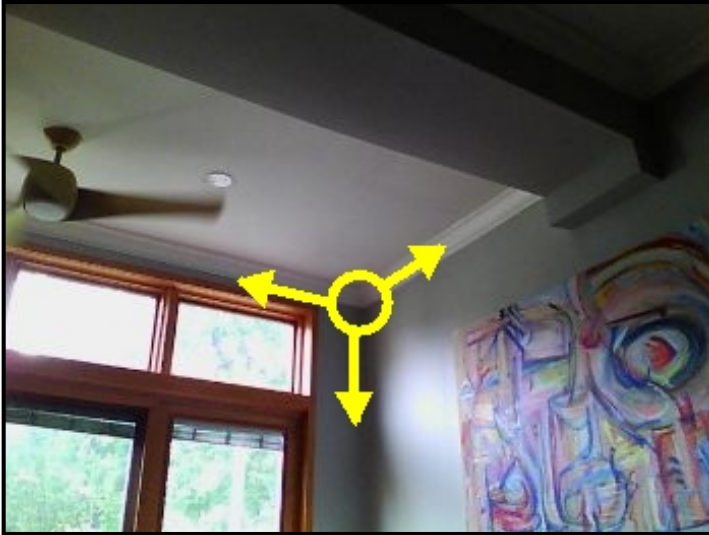
Water entry into corner wall/ceiling area.
