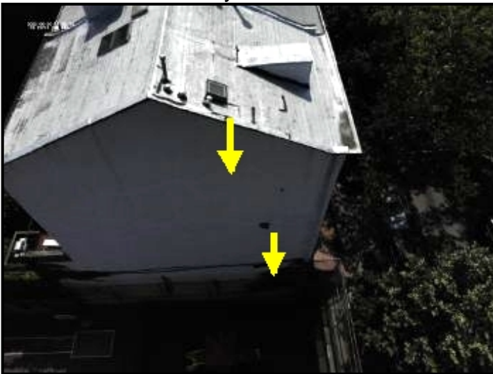
Water entering through roof membrane/parapet wall coping stone connection point, cascading down through the side facade and depositing into the internal wall areas below.
