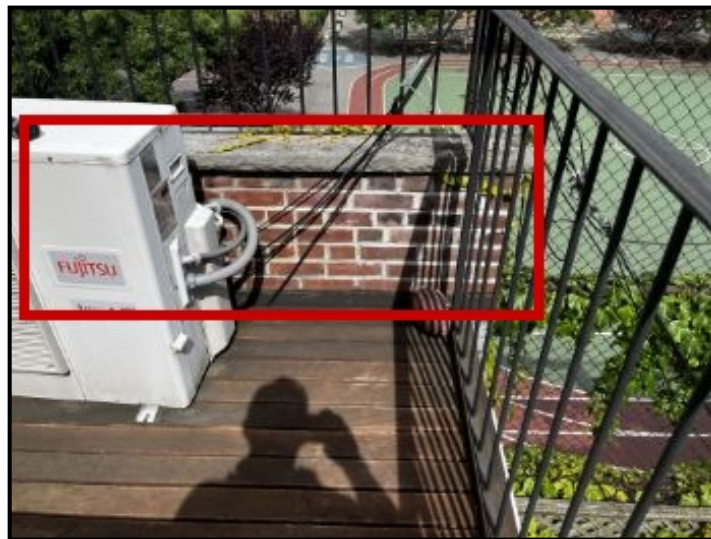
Repair Point: Waterproof inner and outer parapet wall brick system. Install aluminum flashing cap over parapet wall coping stone.
