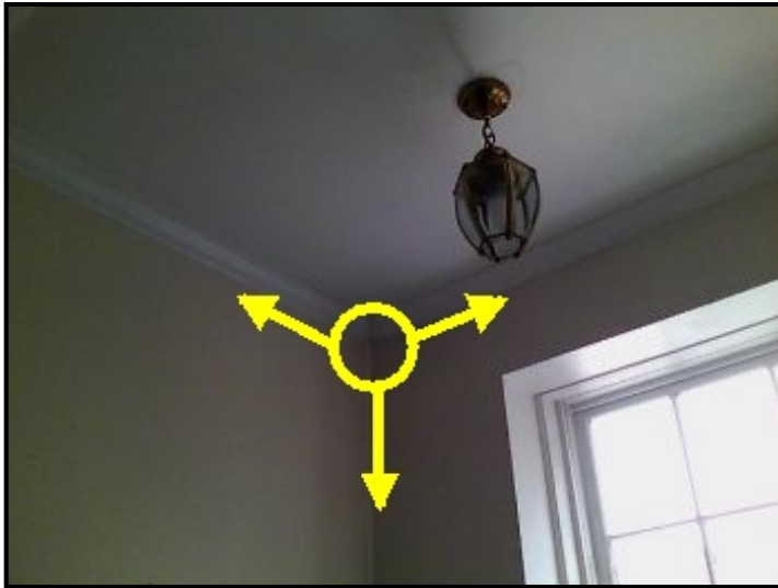
Severe water entry into corner wall area.
