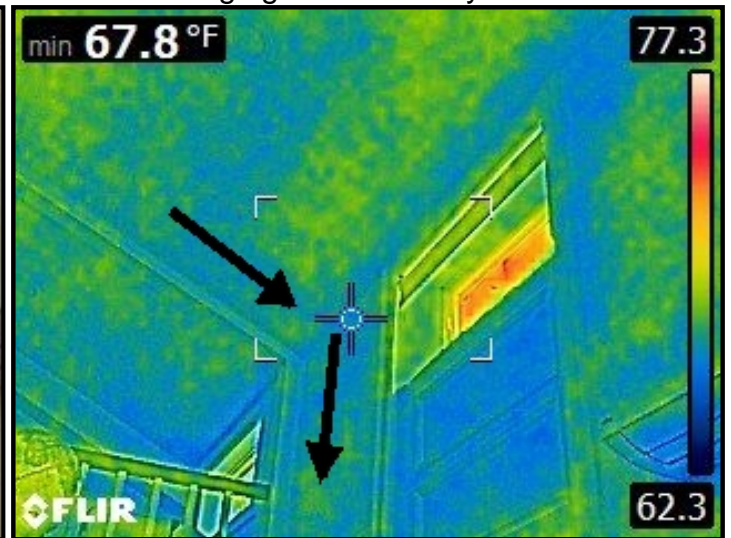
Infrared imaging of water entry into ceiling/wall area.
