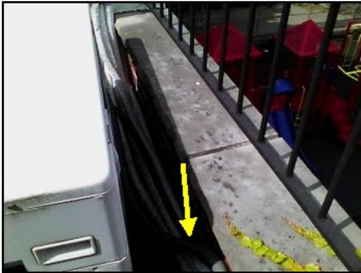
Water entering through parapet wall coping stone system and cascading down into the ceiling/wall area below.
