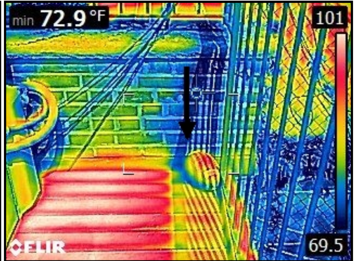
Infrared imaging of water entering through parapet wall and cascading down into the ceiling/wall area below.
