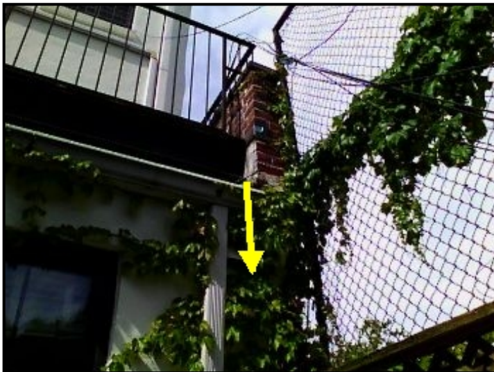
Water entering through parapet wall and cascading down into the ceiling/wall area below.
