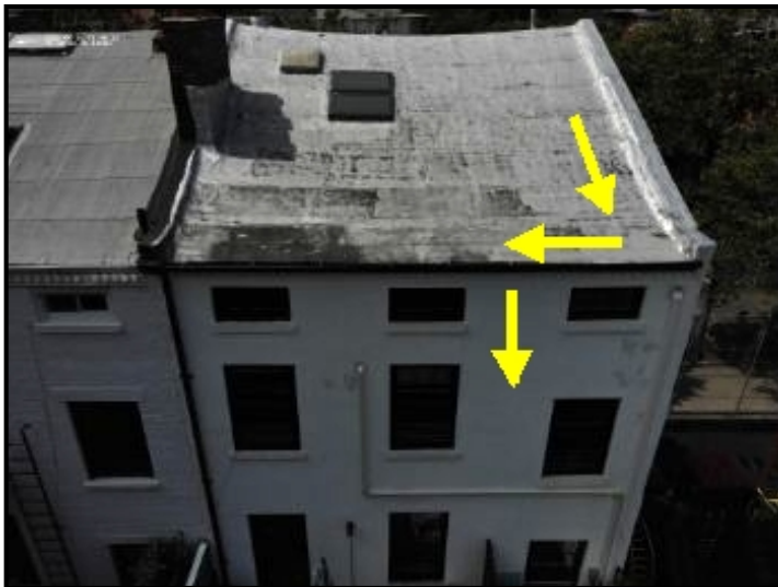
Water entering through the roof membrane system and cascading down into the rear facade.
