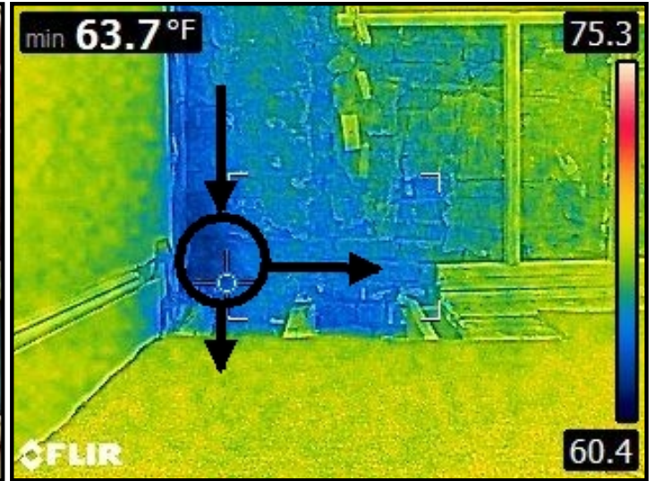
Infrared imaging of water cascading down through wall area.
