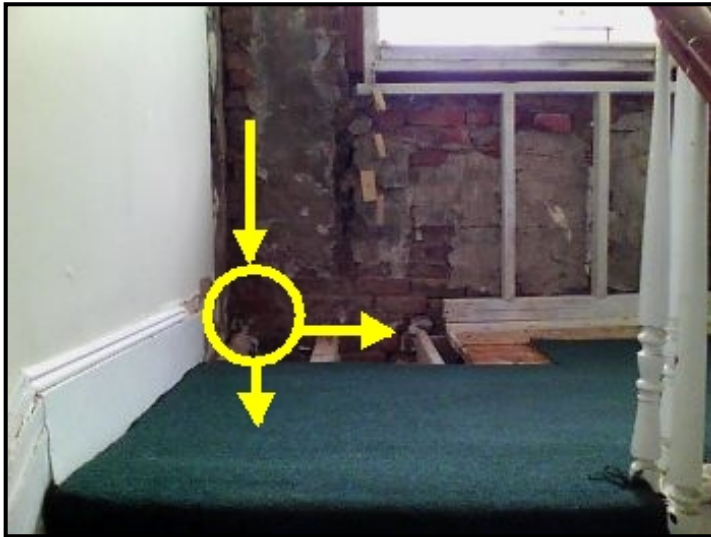
Water cascading down through wall area.
