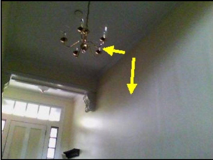
Water entry into wall area.
