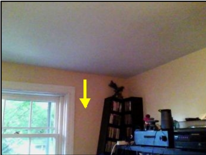
Water entry into wall/ceiling area.
