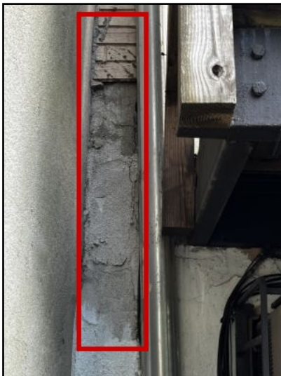
Repair Point: Patch masonry joints. Waterproof area accordingly.
