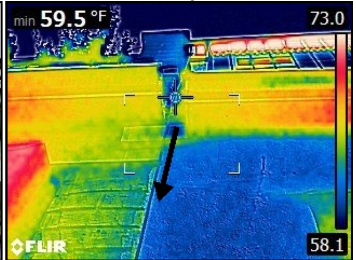
Infrared imaging of water entering through the rear facade between the gutter trays and through the brick parapet wall above.
