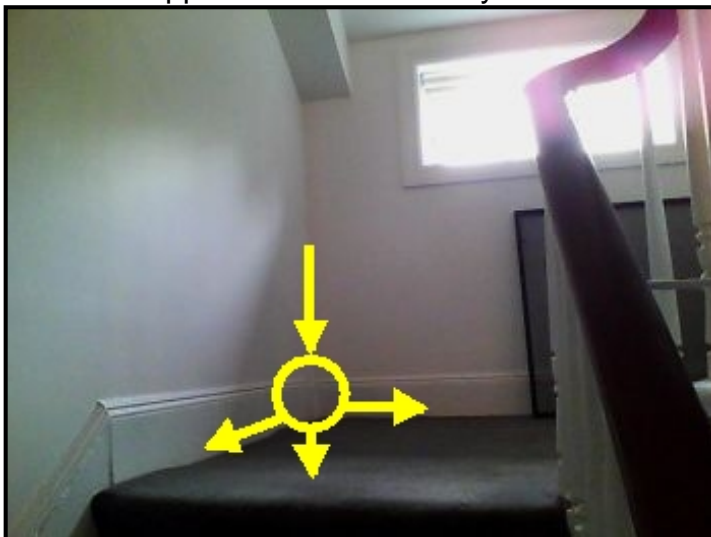
Severe water entry into corner wall area from upper roof membrane system.
