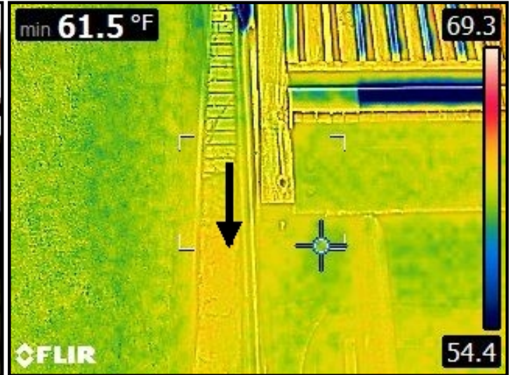
Infrared imaging of water entering through rear facade and backflowing into the internal wall area.
