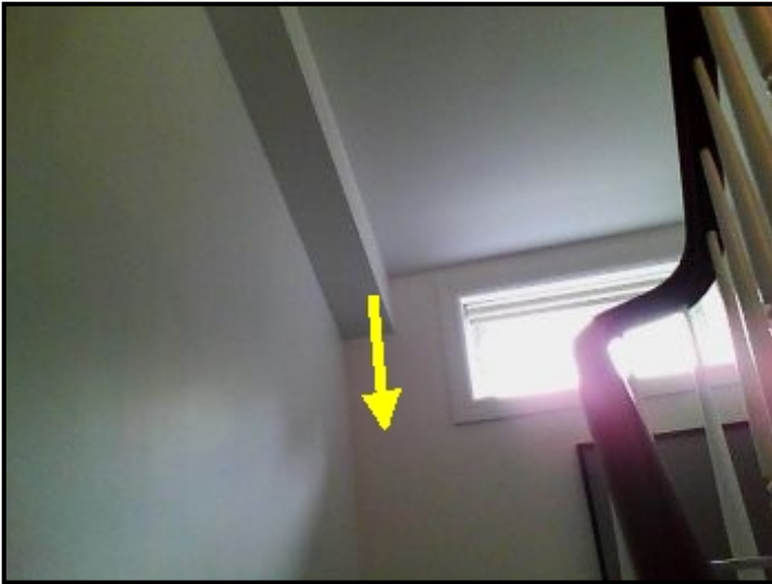
Severe water entry into corner wall area from upper roof membrane system.
