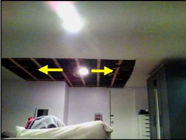
Water entry into ceiling area.
