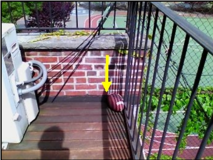
Water entering through parapet wall and cascading down into the ceiling/wall area below.
