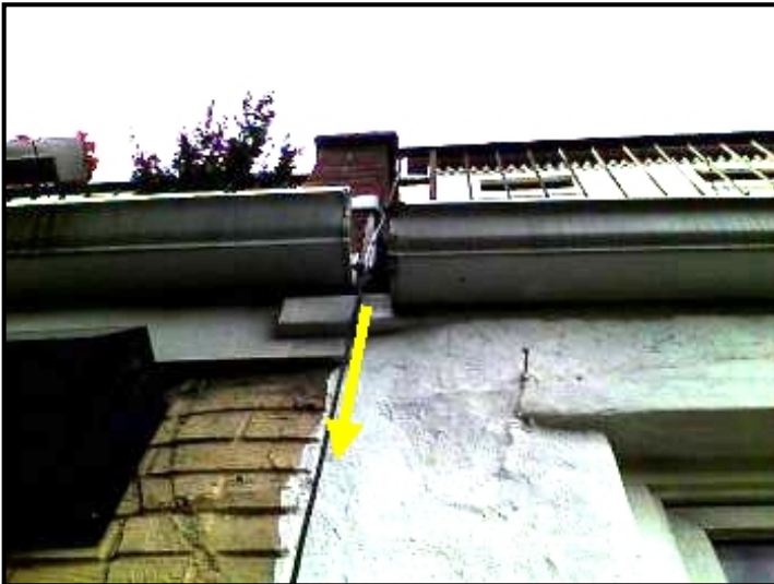
Water entering through the rear facade between the gutter trays and through the brick parapet wall above.
