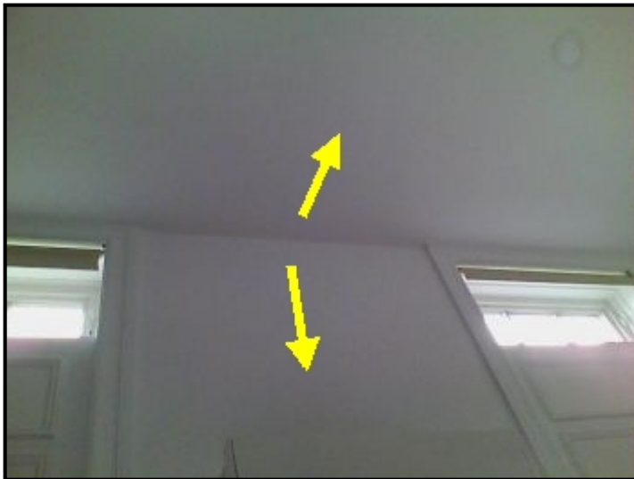
Water entry into ceiling/wall area.
