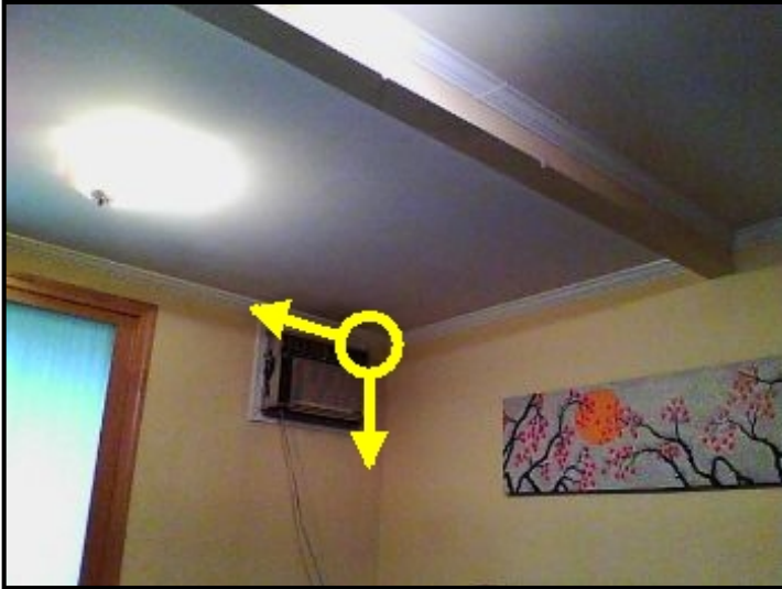
Water entry into corner wall area.
