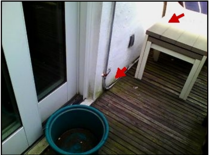
Repair Point: Remove deck planks from around facade. Waterproof area accordingly.
