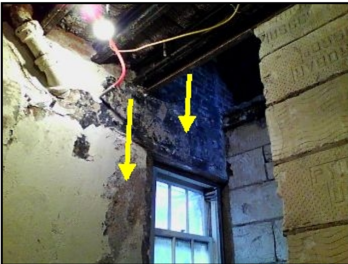
Water entry into wall/window frame area.
