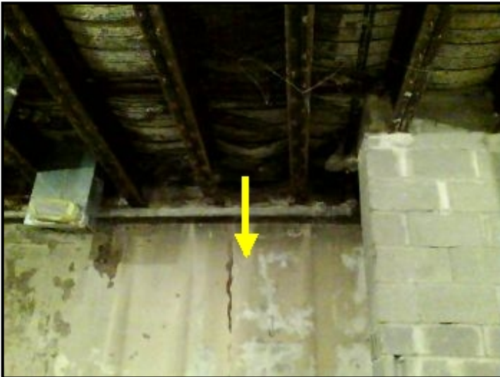
Water entry into wall/ceiling area.
