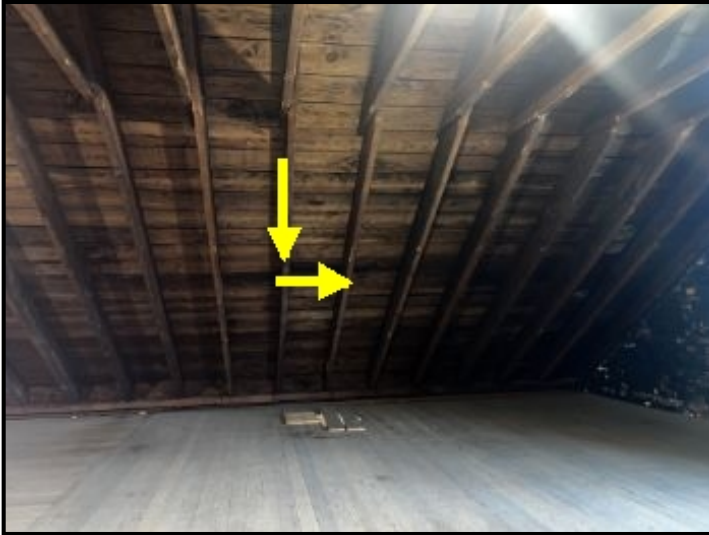
Water entry into attic ceiling.
