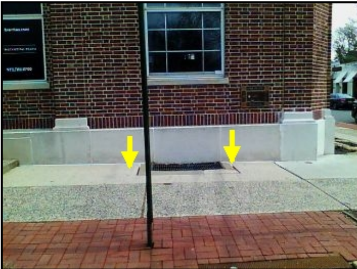
Water entering through sidewalk connection point to brick facade and cascading down into the wall/window frame area below.
