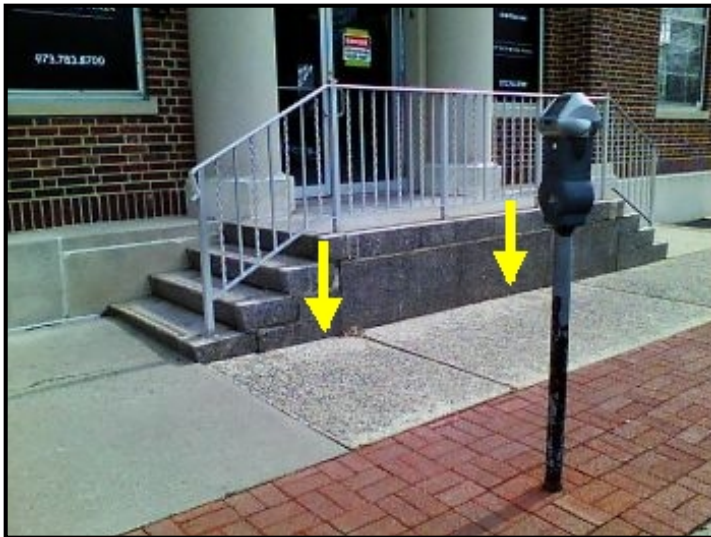
Widespread and severe water entry through the front access stairs/stoop and cascading down into the ceiling/wall area below.
