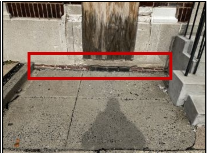
Repair Point: Install new window or close structural opening completely. Seal sidewalk/facade connection point. Conduct followup scans of window bay area below grate.
