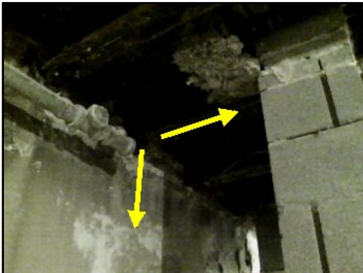
Water entry into wall/ceiling area.
