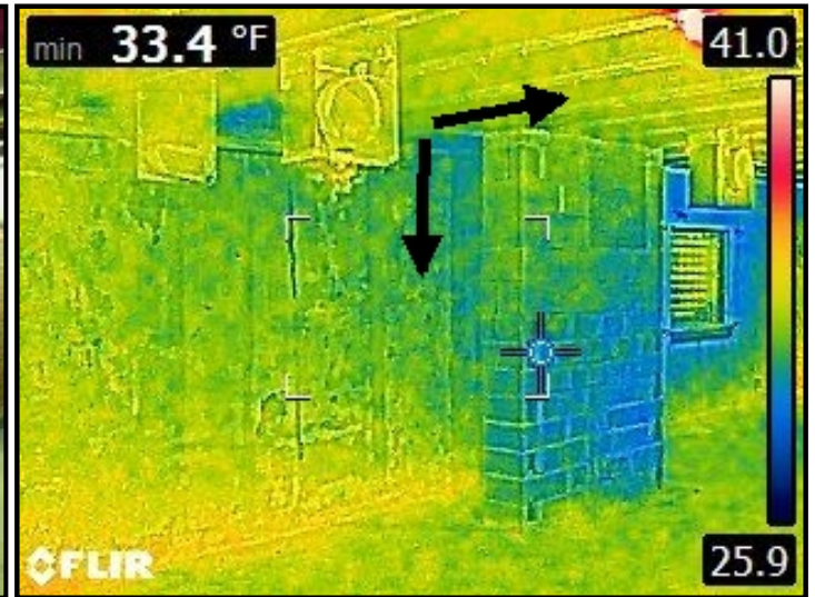
Infrared imaging of water entry into wall/ceiling area.
