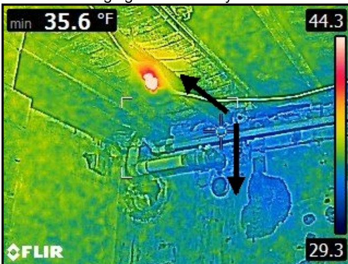
Infrared imaging of water entry into wall area.
