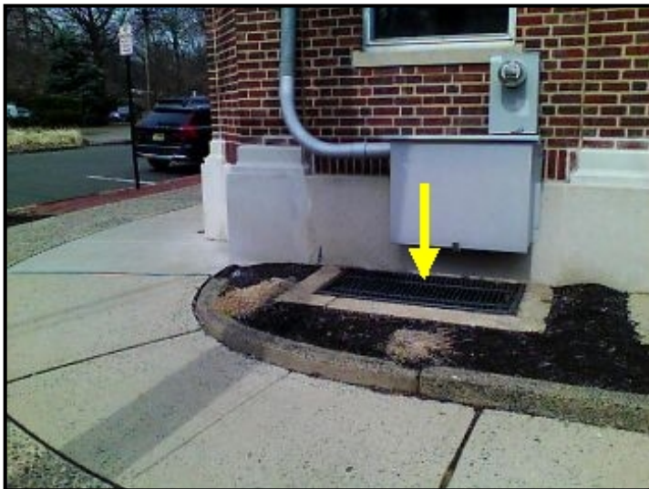
Water entering through utility connection point to brick facade and cascading down into the upper wall/window frame area below.
