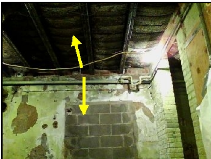
Water entry into wall area.
