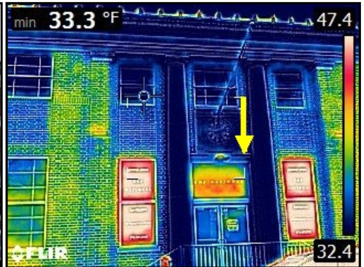
Infrared imaging of water entering through upper brick facade behind pillar and cascading down into the internal wall area below.
