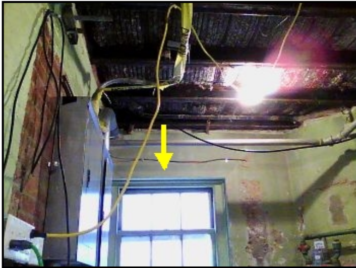
Water entry into wall/window frame area.
