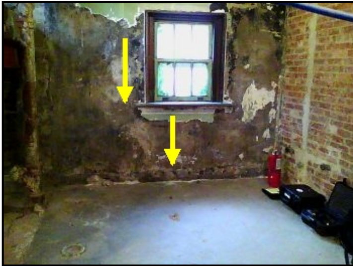
Water entry into wall/window frame area.
