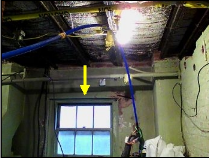
Water entry into wall/window frame area.
