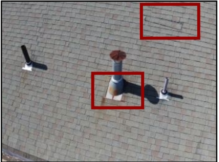
Repair Point: Replace shingles. Inspect area around roof vent and waterproof as needed.
