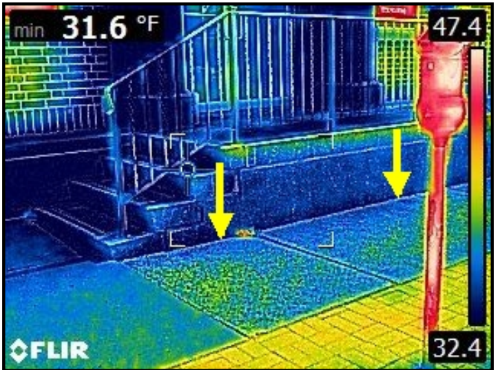
Infrared imaging of widespread and severe water entry through the front access stairs/stoop and cascading down into the ceiling/wall area below.
