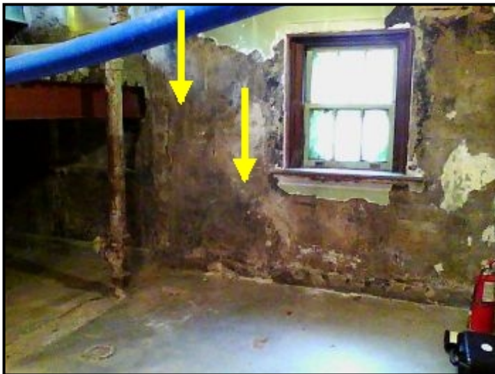
Water entry into wall/window frame area.
