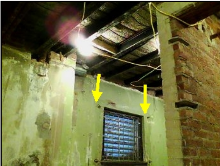
Water entry into wall/window frame area.
