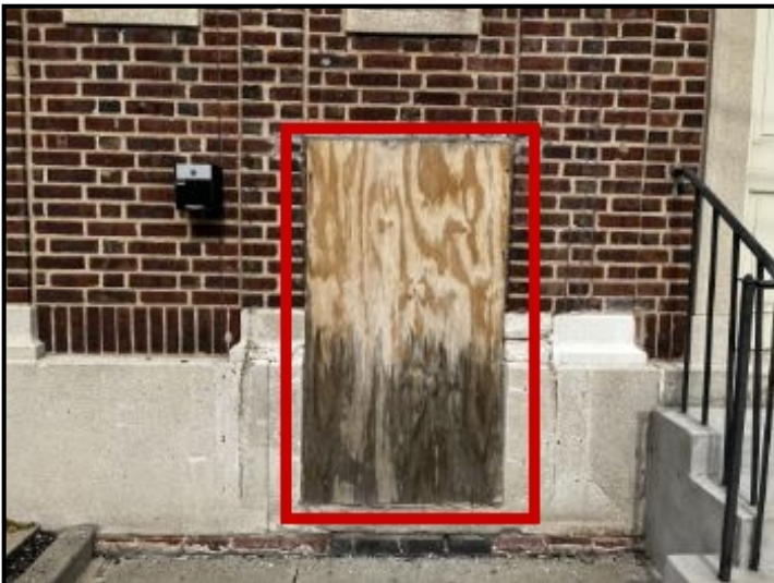
Repair Point: Install new window or close structural opening completely. Seal sidewalk/facade connection point. Conduct followup scans of window bay area below grate.
