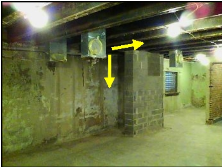
Water entry into wall/ceiling area.
