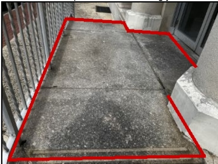
Repair Point: Remove all tile from stairs/stoop. Waterproof area accordingly.
