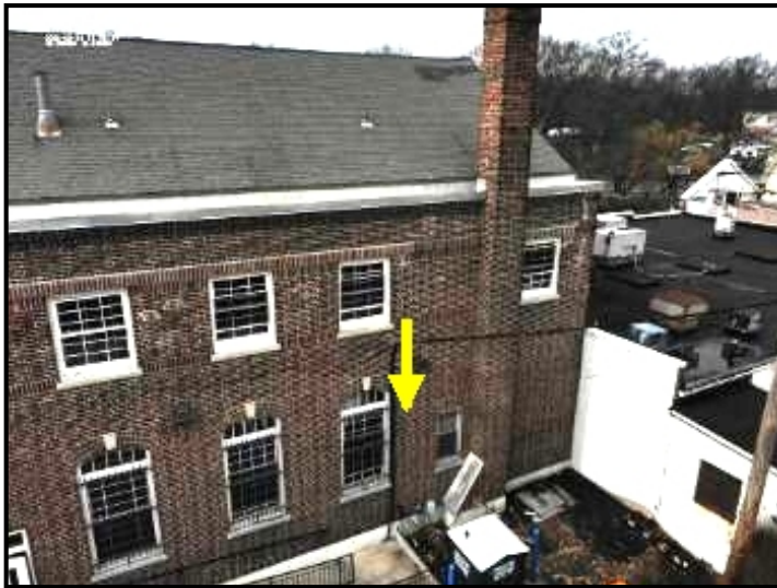
Water entering through brick facade and cascading down into the wall area below.
