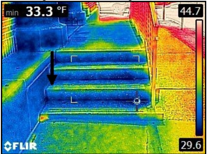
Infrared imaging of widespread and severe water entry through the front access stairs/stoop and cascading down into the ceiling/wall area below.
