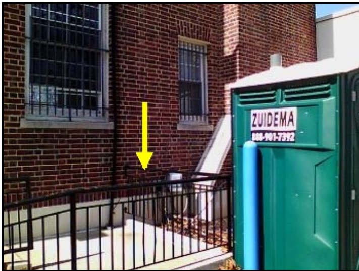
Water entering through brick facade and cascading down into the wall area below.
