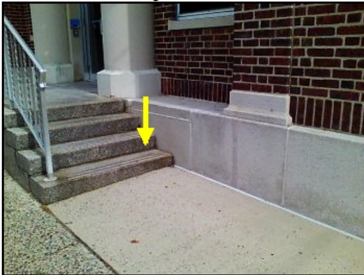
Widespread and severe water entry through the front access stairs/stoop and cascading down into the ceiling/wall area below.
