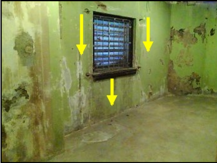
Water entry into wall/window frame area.
