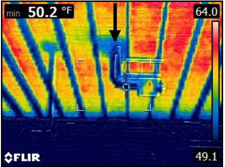
Infrared imaging of water entry into attic ceiling around vent line.
