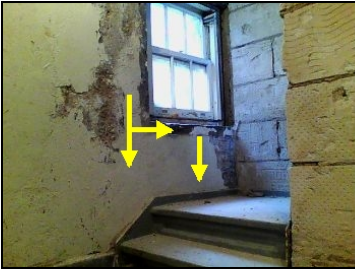
Water entry into wall/window frame area.
