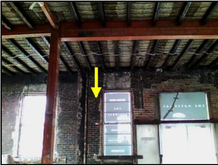
Water entry into upper wall area.
