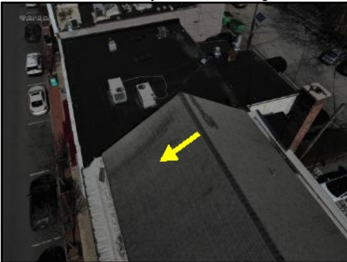
Water entering through roof peak shingles and cascading down into the attic ceiling area below.
