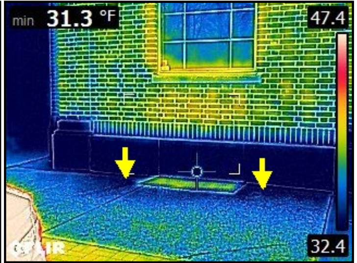
Infrared imaging of water entering through sidewalk/brick facade connection point and cascading down into the wall/window frame area below.
