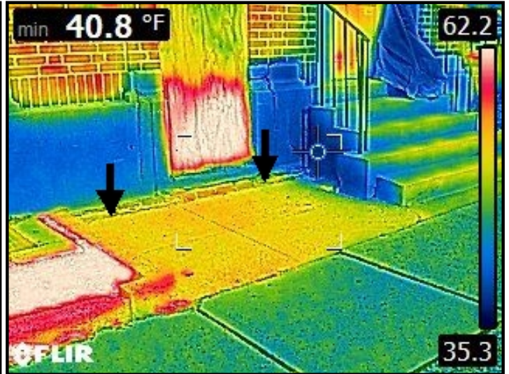
Infrared imaging of water entering through sidewalk connection point to facade and cascading down into the wall area below.
