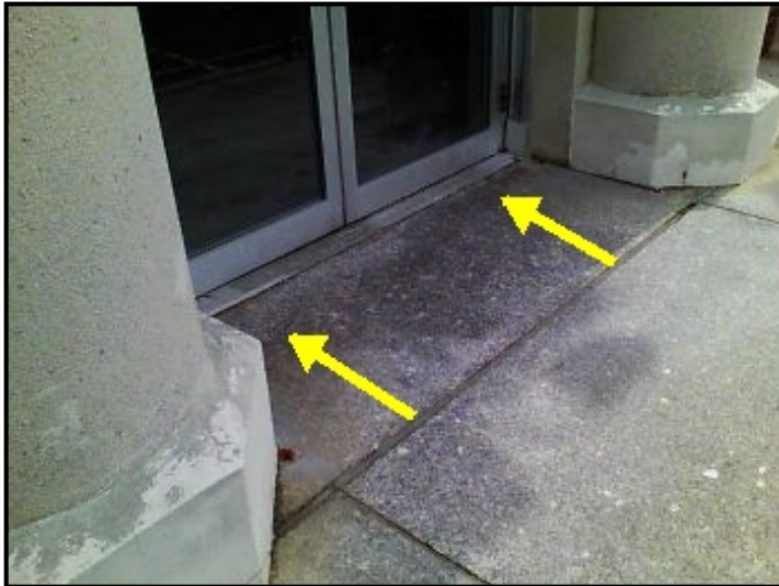
Widespread and severe water entry through the front access stairs/stoop and cascading down into the ceiling/wall area below.
