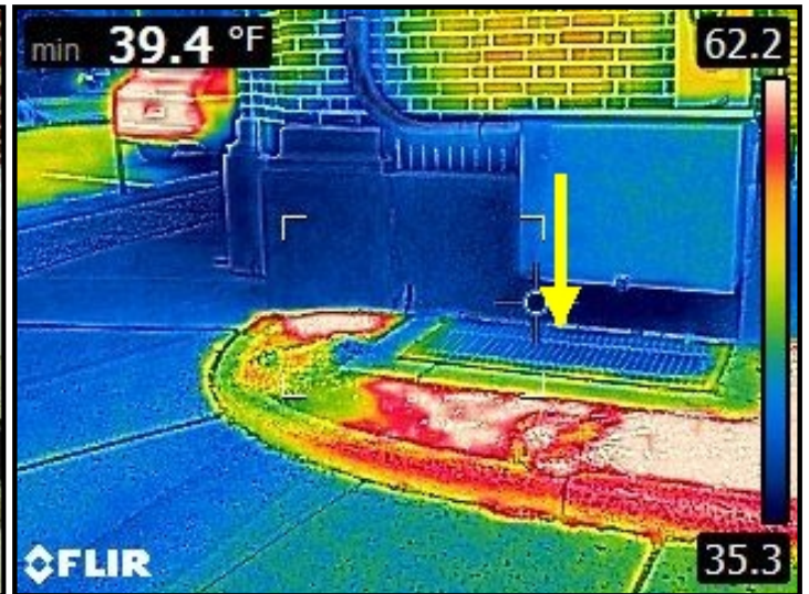
Infrared imaging of water entering through utility connection point to brick facade and cascading down into the upper wall/window frame area below.
