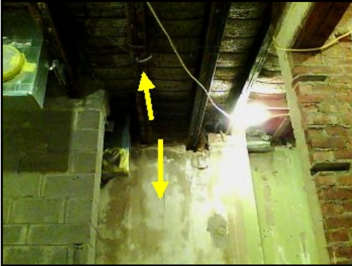
Water entry into wall/ceiling area.
