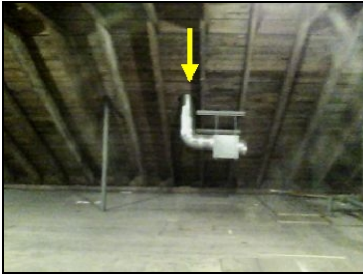
Water entry into attic ceiling around vent line.
