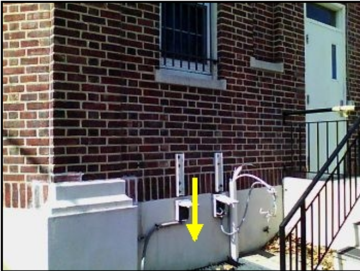
Water entering through brick facade and cascading down into wall/window frame area below.
