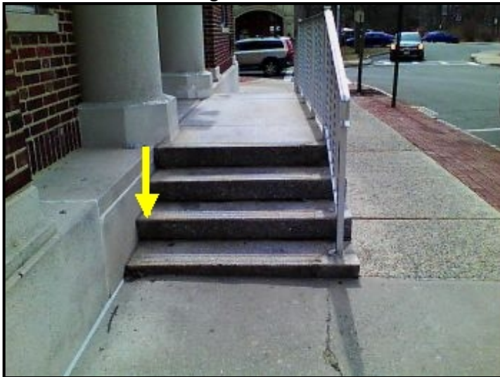
Widespread and severe water entry through the front access stairs/stoop and cascading down into the ceiling/wall area below.
