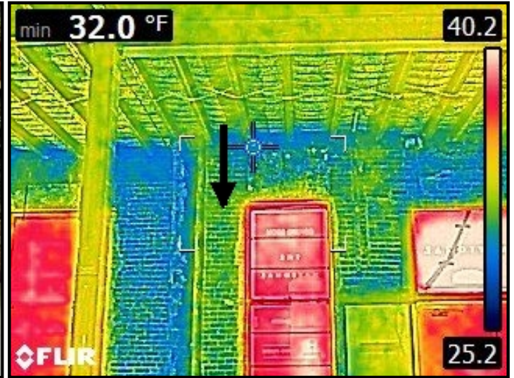
Infrared imaging of water entry into upper wall area.
