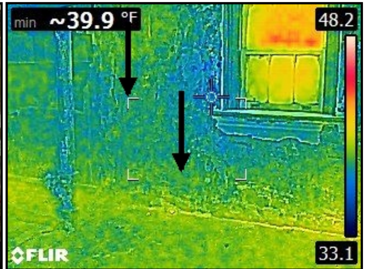
Infrared imaging of water entry into wall/window frame area.
