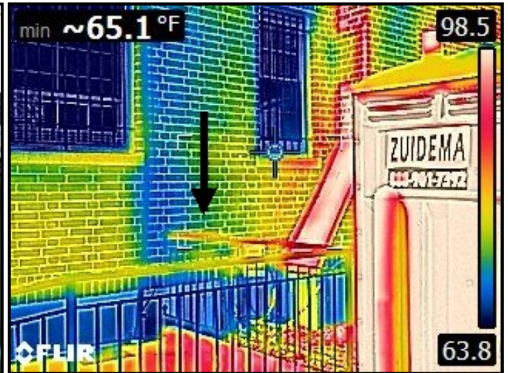
Infrared imaging of water entering through brick facade and cascading down into the wall area below.
