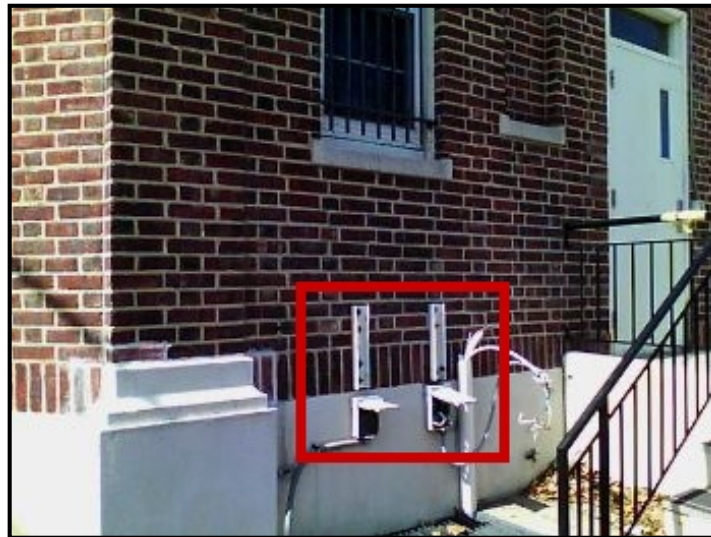
Repair Point: Seal around utility connection points to facade. Remove window bay grate and conduct followup scans of the area.
