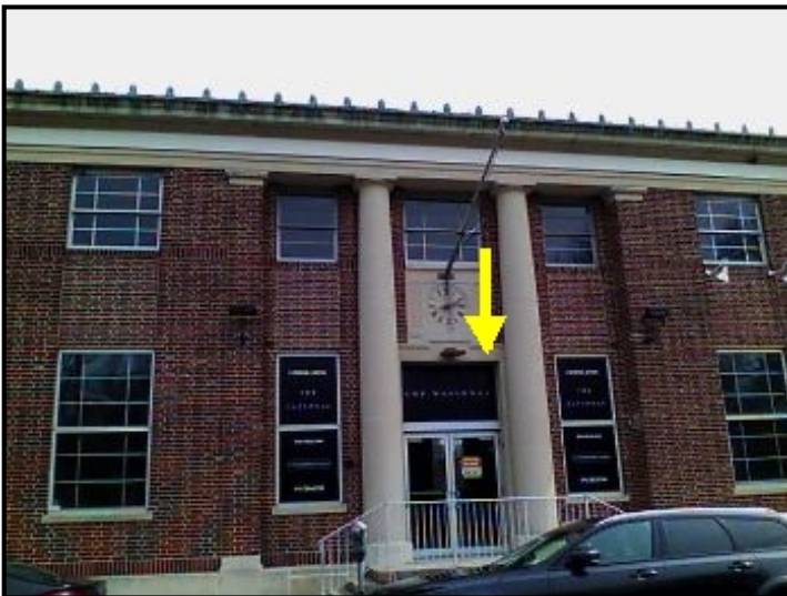
Water entering through upper brick facade behind pillar and cascading down into the internal wall area below.
