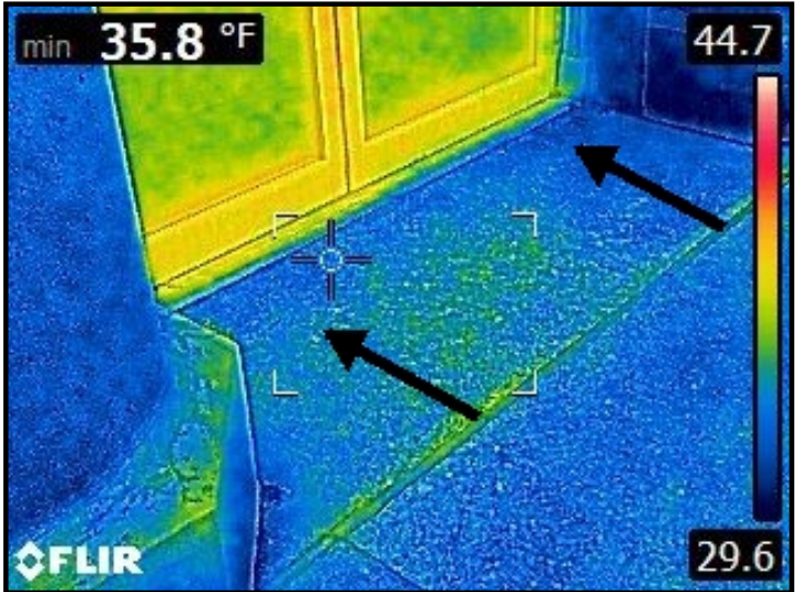
Infrared imaging of widespread and severe water entry through the front access stairs/stoop and cascading down into the ceiling/wall area below.
