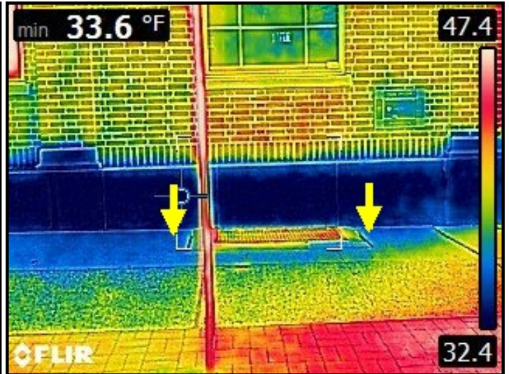
Infrared imaging of water entering through sidewalk connection point to brick facade and cascading down into the wall/window frame area below.
