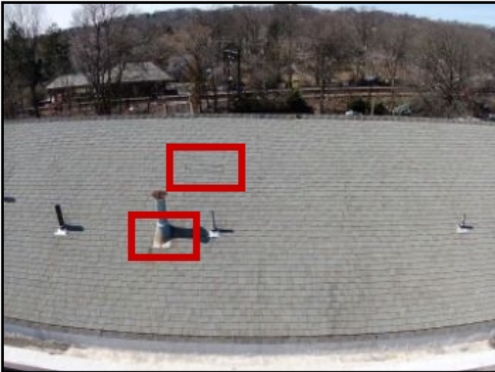
Repair Point: Replace shingles. Inspect area around roof vent and waterproof as needed.
