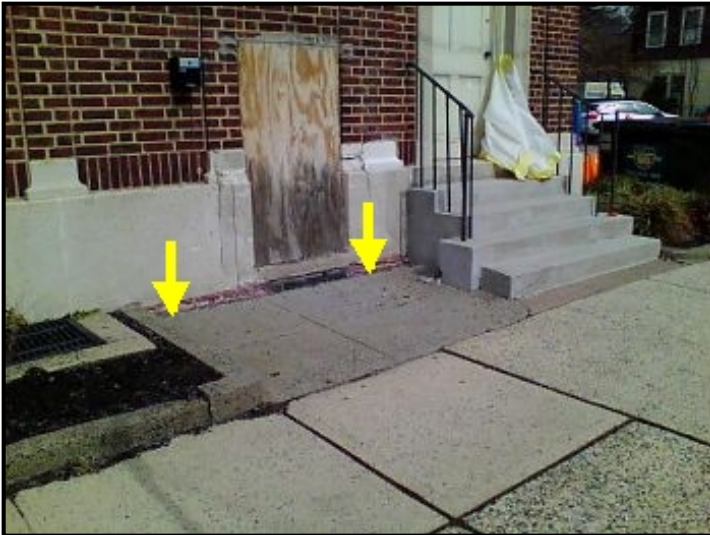
Water entering through sidewalk connection point to facade and cascading down into the wall area below.
