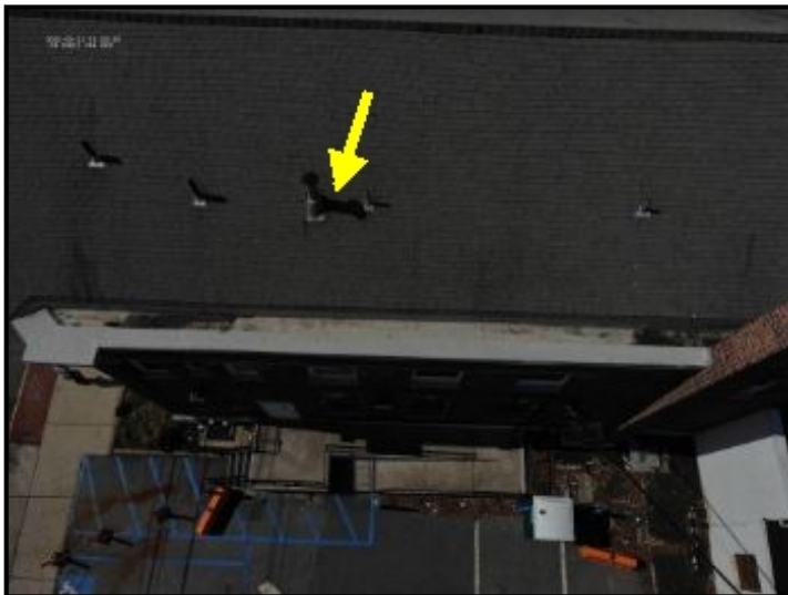
Water entering through shingle roof system, cascading down and depositing around the roof vent/internal ceiling area below.
