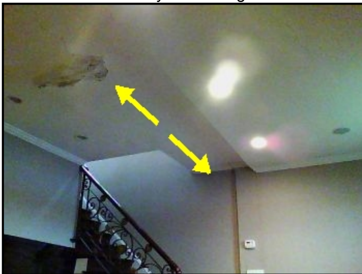
Water entry into ceiling area.
