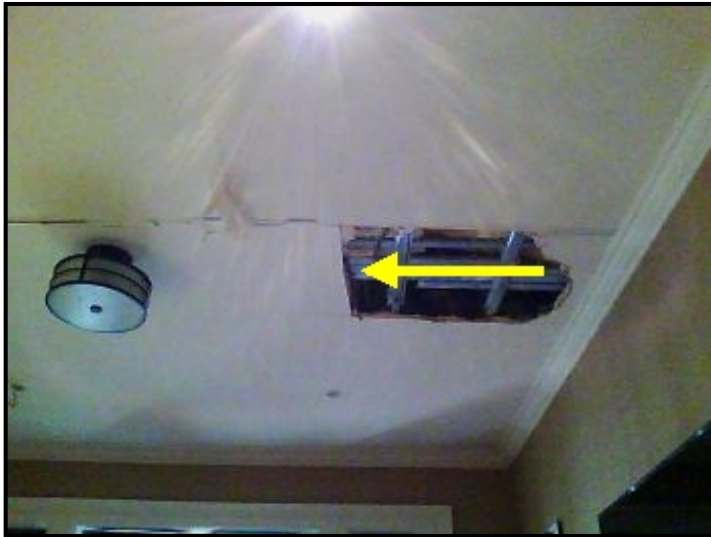
Water entry into ceiling area.
