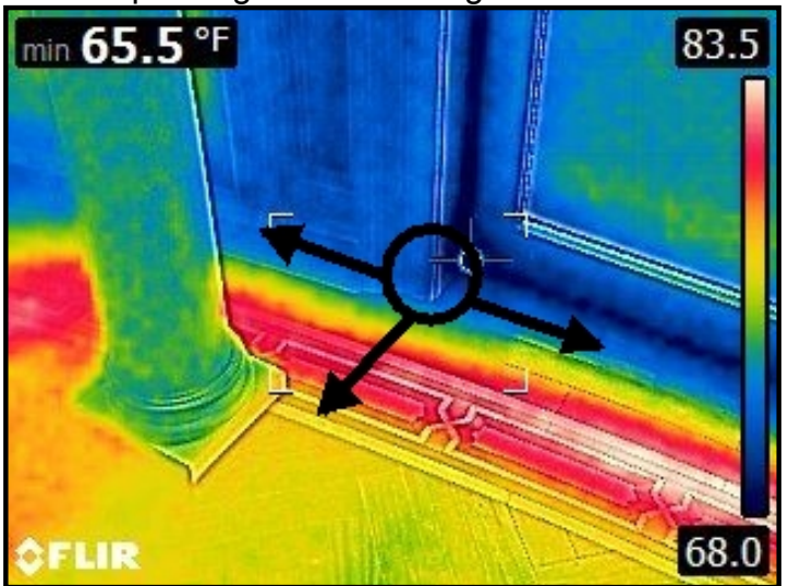
Infrared imaging of water entering through terrace tile and door baseplate, cascading down and depositing into the ceiling areas below.
