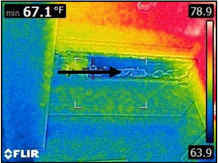
Infrared imaging of water entry into ceiling area.
