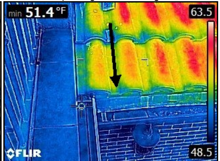
Infrared imaging of water entering through broken spanish roof tile, cascading down and depositing into the brick facade eventually entering into the ceiling area below.
