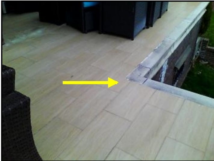
Water cascading out through the tile system, depositing into the brick facade and cascading down into the ceiling area below.
