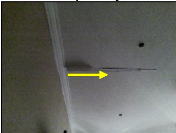
Water entry into ceiling area.
