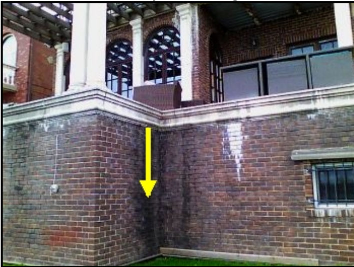
Water entering through brick facade, backflowing into the substrate and depositing into the ceiling area below.
