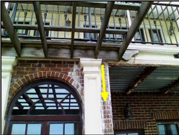
Severe water entry into brick facade and cascading down into the ceiling area below.
