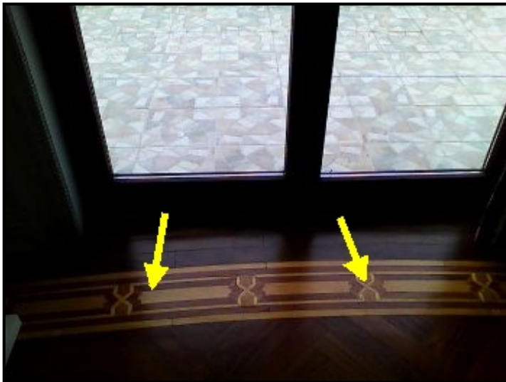
Water entering through terrace tile and door baseplate, cascading down and depositing into the ceiling areas below.
