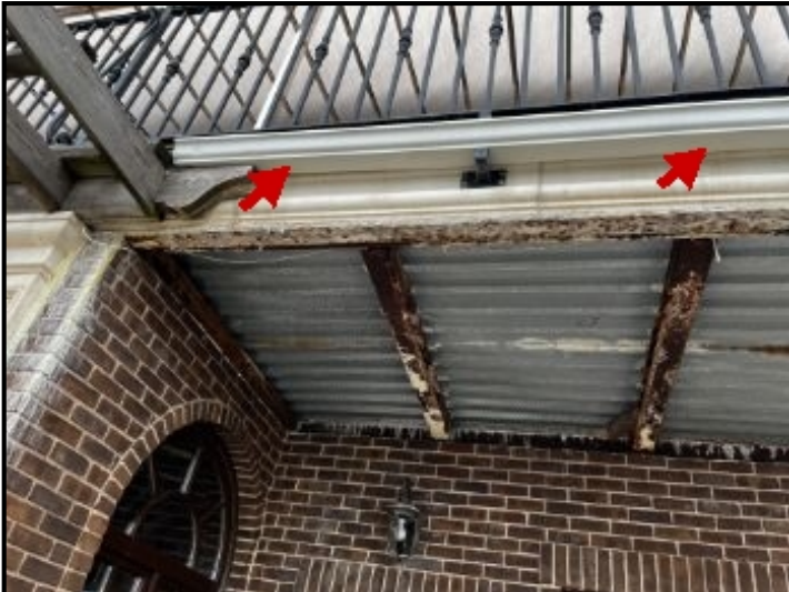
Repair Point: Remove wood pavilion from facade. Remove gutter system. Waterproof area accordingly.
