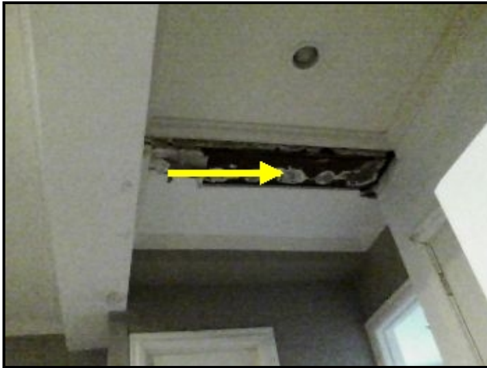
Water entry into ceiling area.
