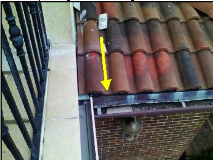
Water entering through broken spanish roof tile, cascading down and depositing into the brick facade eventually entering into the ceiling area below.
