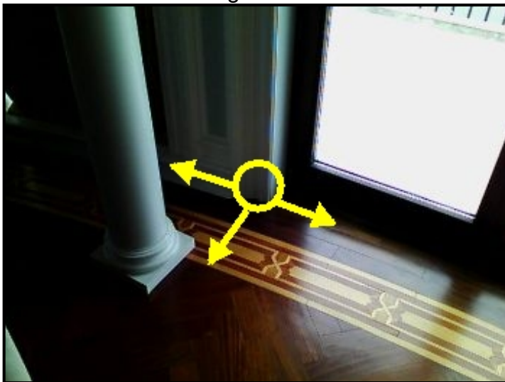
Water entering through terrace tile and door baseplate, cascading down and depositing into the ceiling areas below.
