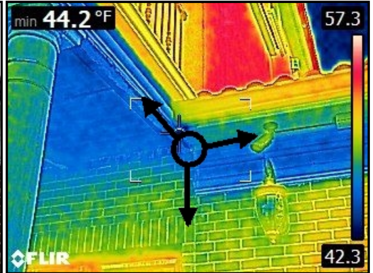
Infrared imaging of water cascading down through brick and depositing into the ceiling area below.
