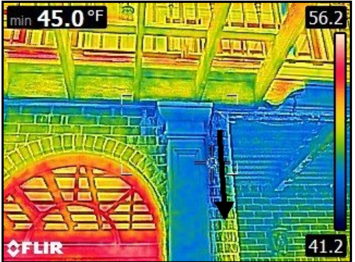
Infrared imaging of severe water entry into brick facade and cascading down into the ceiling area below.
