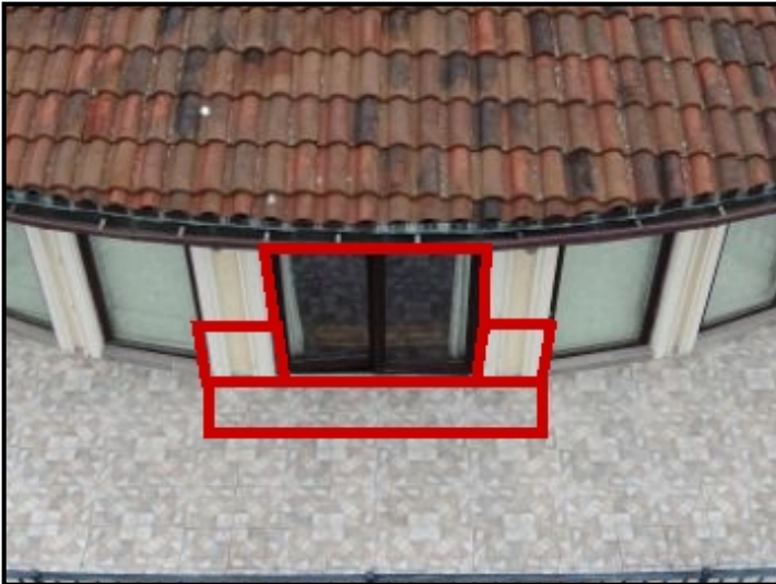
Repair Point: Excavate tile around door baseplate and EIFS facade. Remove door frame entirely. Waterproof and flash area accordingly.
