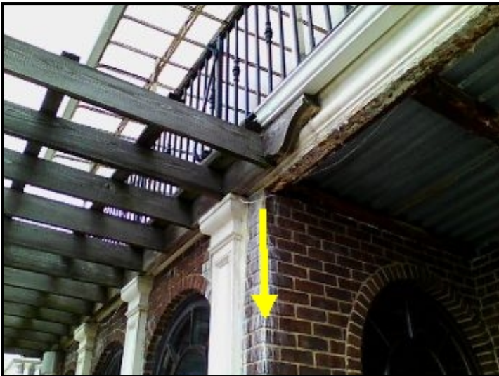
Severe water entry into brick facade and cascading down into the ceiling area below.
