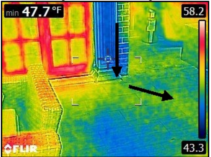
Infrared imaging of water cascading down through brick facade and depositing into the tile floor eventually entering into the ceiling area below.
