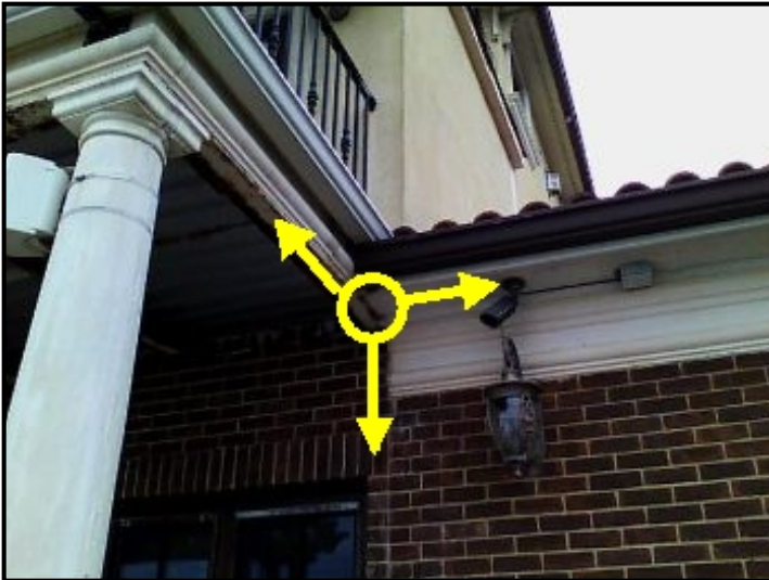
Water cascading down through brick and depositing into the ceiling area below.
