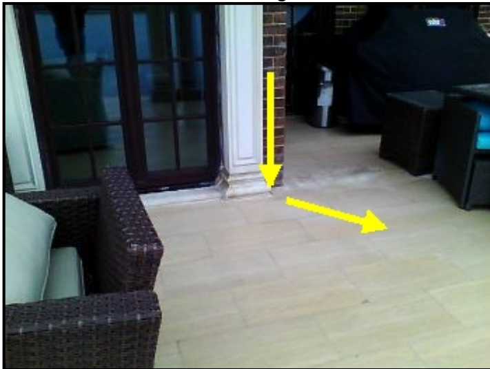
Water cascading down through brick facade and depositing into the tile floor eventually entering into the ceiling area below.
