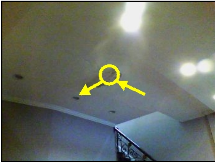
Water entry into ceiling area.
