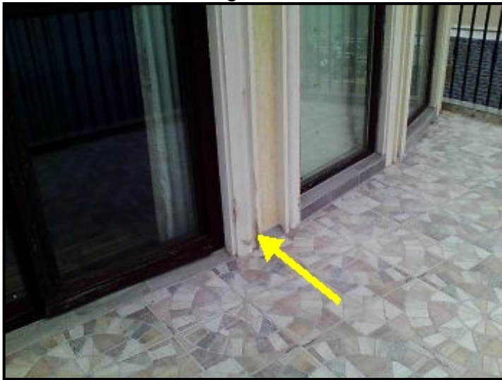
Water entering through terrace tile and door baseplate, cascading down and depositing into the ceiling areas below.
