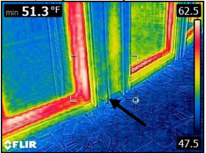
Infrared imaging of water entering through terrace tile and door baseplate, cascading down and depositing into the ceiling areas below.
