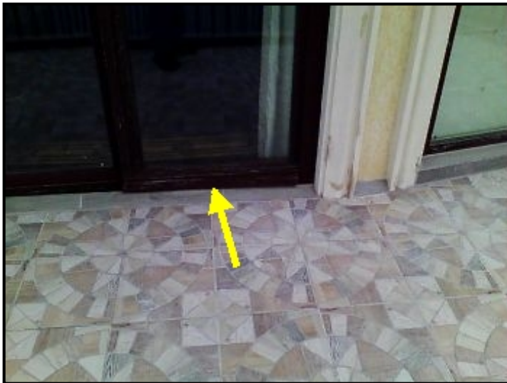
Water entering through terrace tile and door baseplate, cascading down and depositing into the ceiling areas below.
