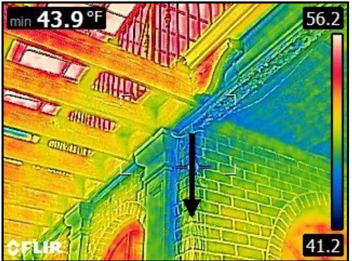
Infrared imaging of severe water entry into brick facade and cascading down into the ceiling area below.
