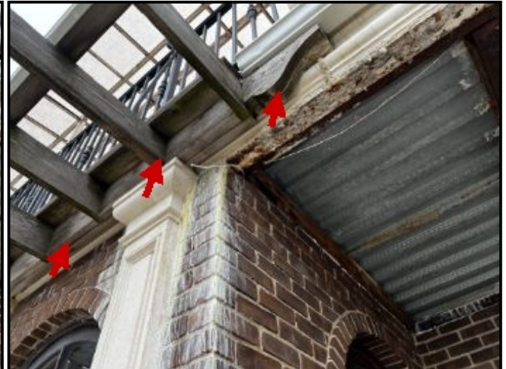
Repair Point: Remove wood pavilion from facade. Remove gutter system. Waterproof area accordingly.
